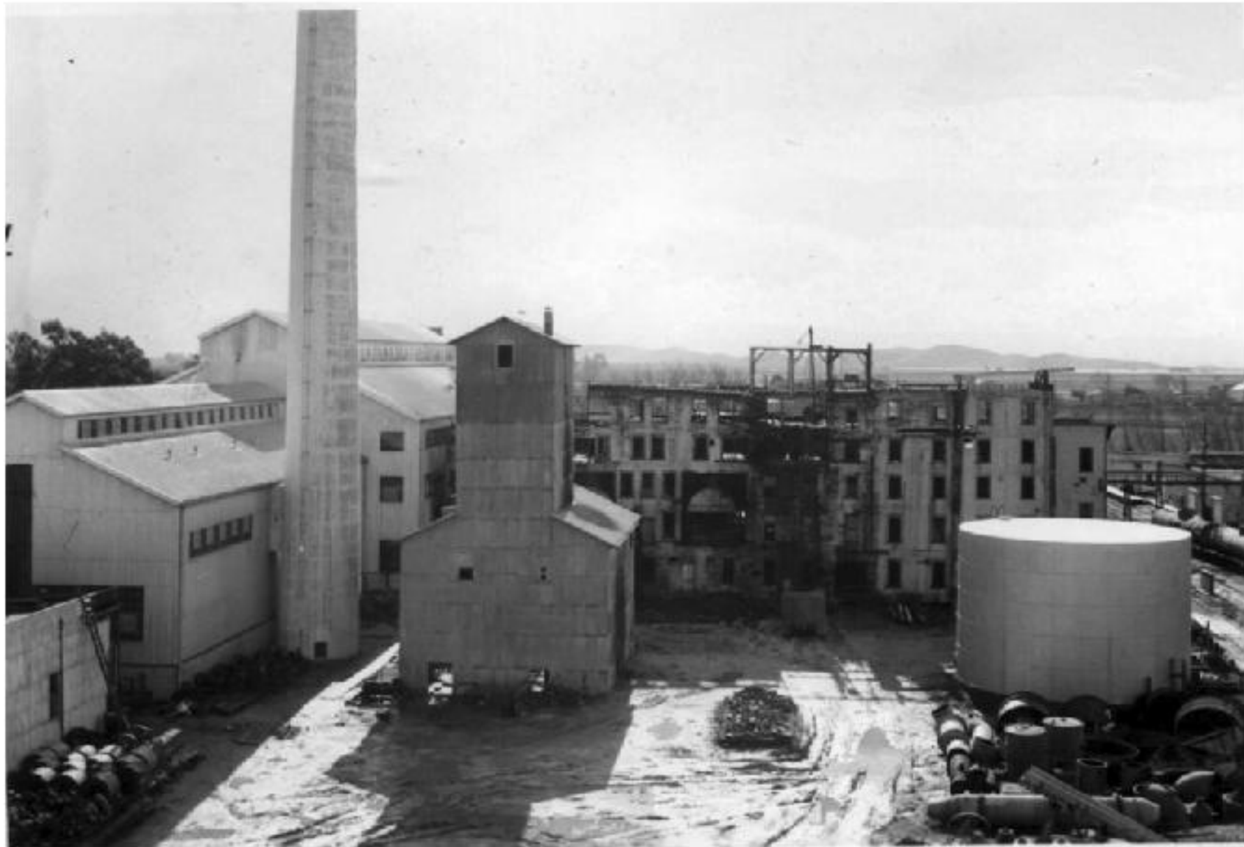
The new building with the signature "Holly" smokestack completed. The old building is in the process of demolition in the background.
