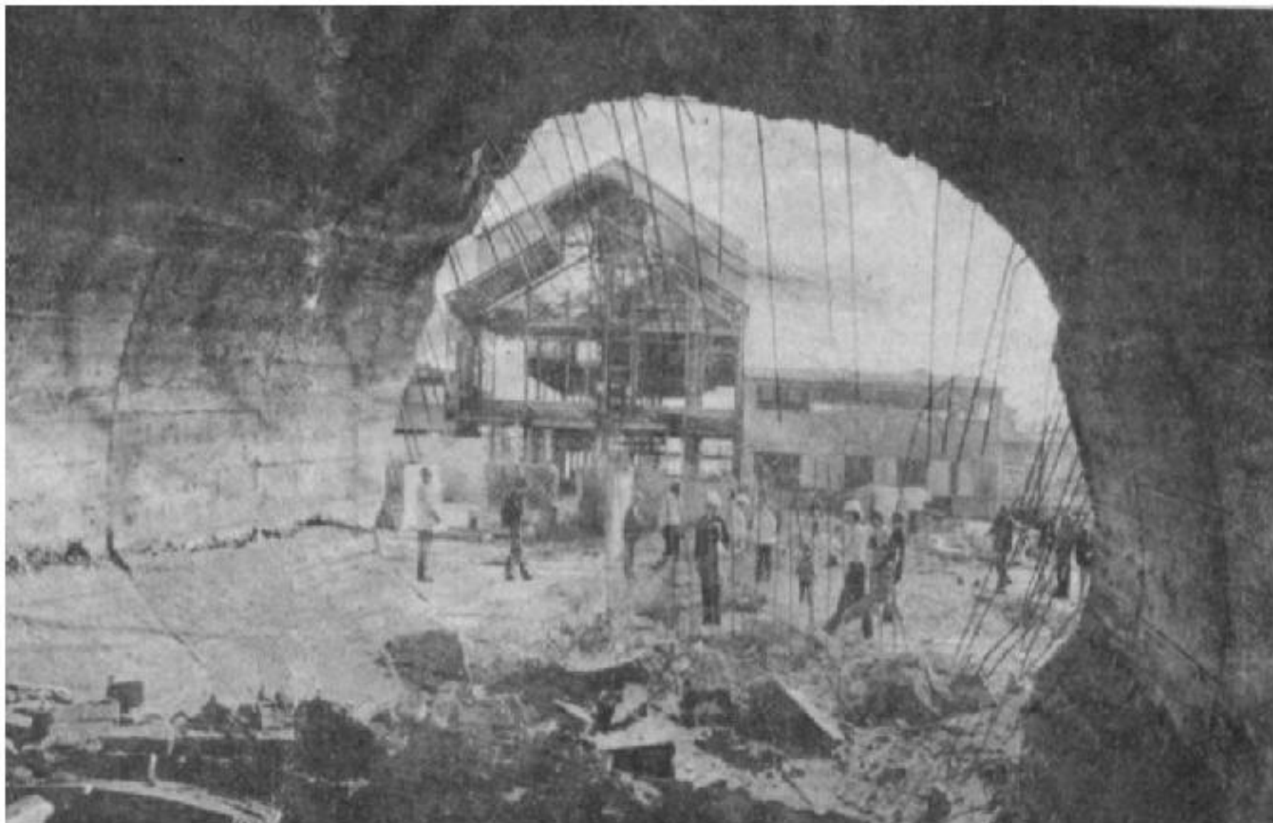
The inside of the Holly Sugar smoke stack showing the old main building in the process of being dismantled. This was the end of the line for Alvarado's sugar mill. Holly's Tracy plant continued to operate until December 2000 after passing through the hands of the Imperial Sugar Company and others before buyers could not be located to keep the mill running. Much of the land that was the mill's is now the city's Legacy Fields sports complex.
