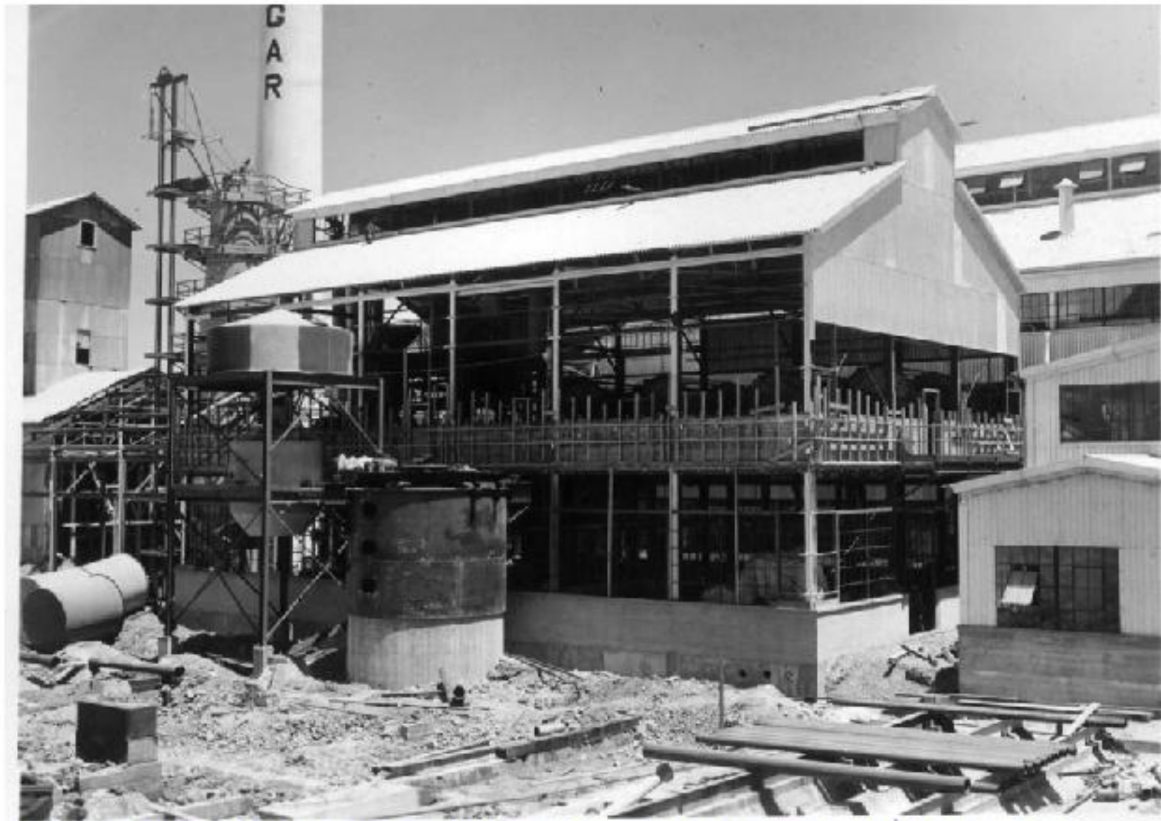
Continuing the renovation with another new building. Nearing completion of the job.
