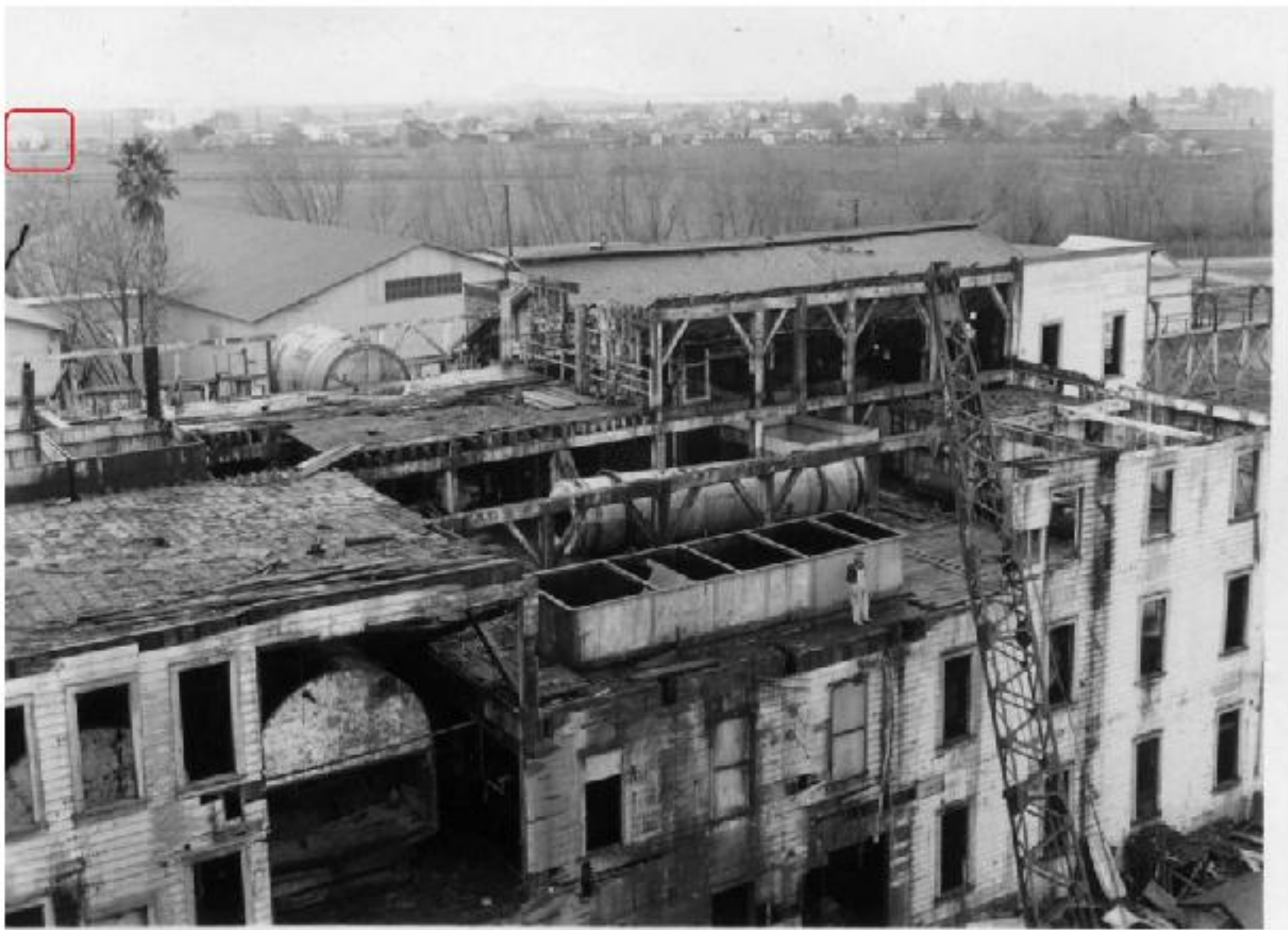
The old structure partially torn down. This photo taken from the east and shooting west shows the branches of the trees of the Alameda Creek behind the building and the town of Alvarado in the distance. To give a proper perspective I have outlined the Alvarado Grammar School on Smith street in red in the upper left.
